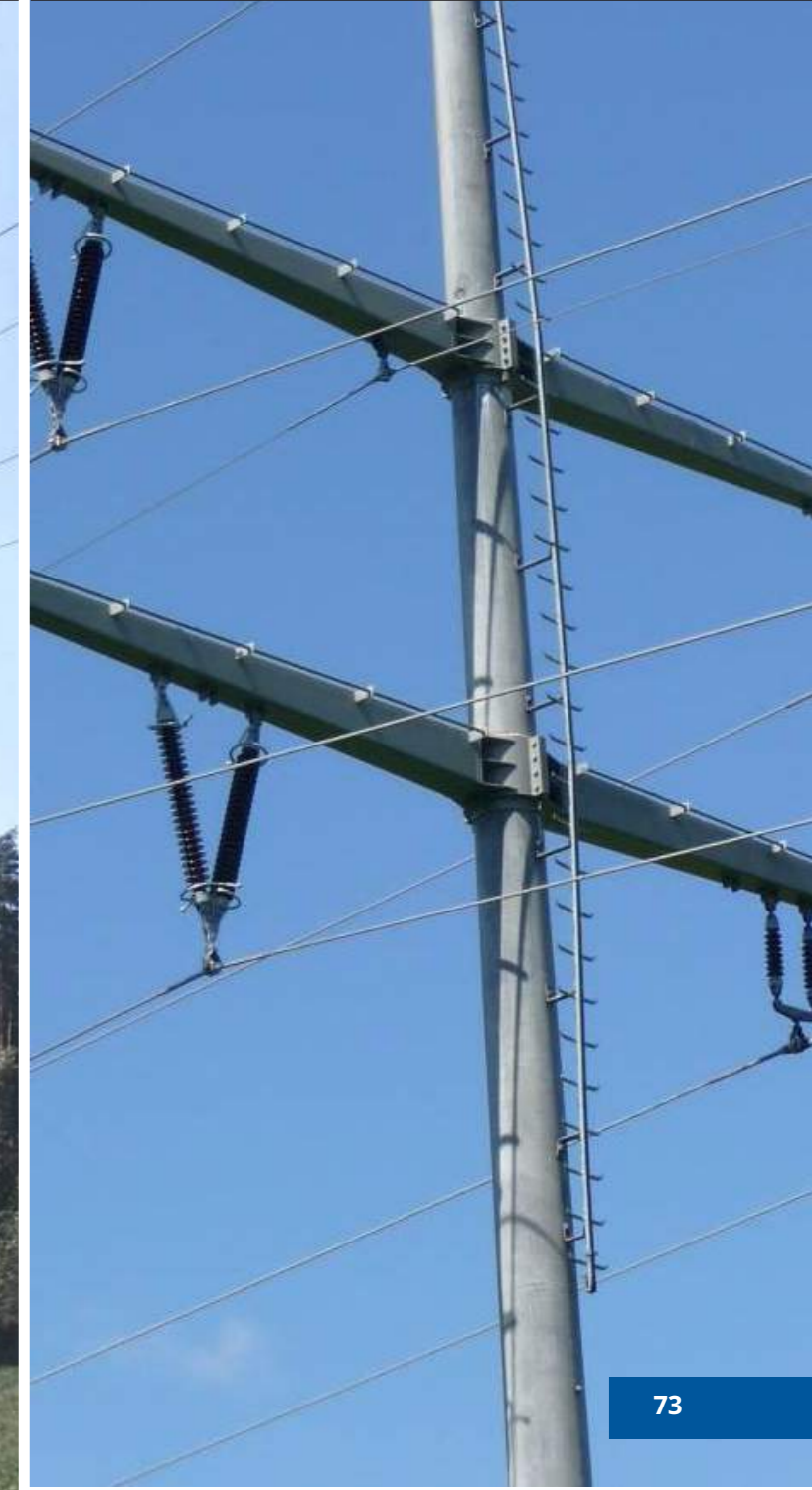
Concrete Pole with Steel Crossarm
