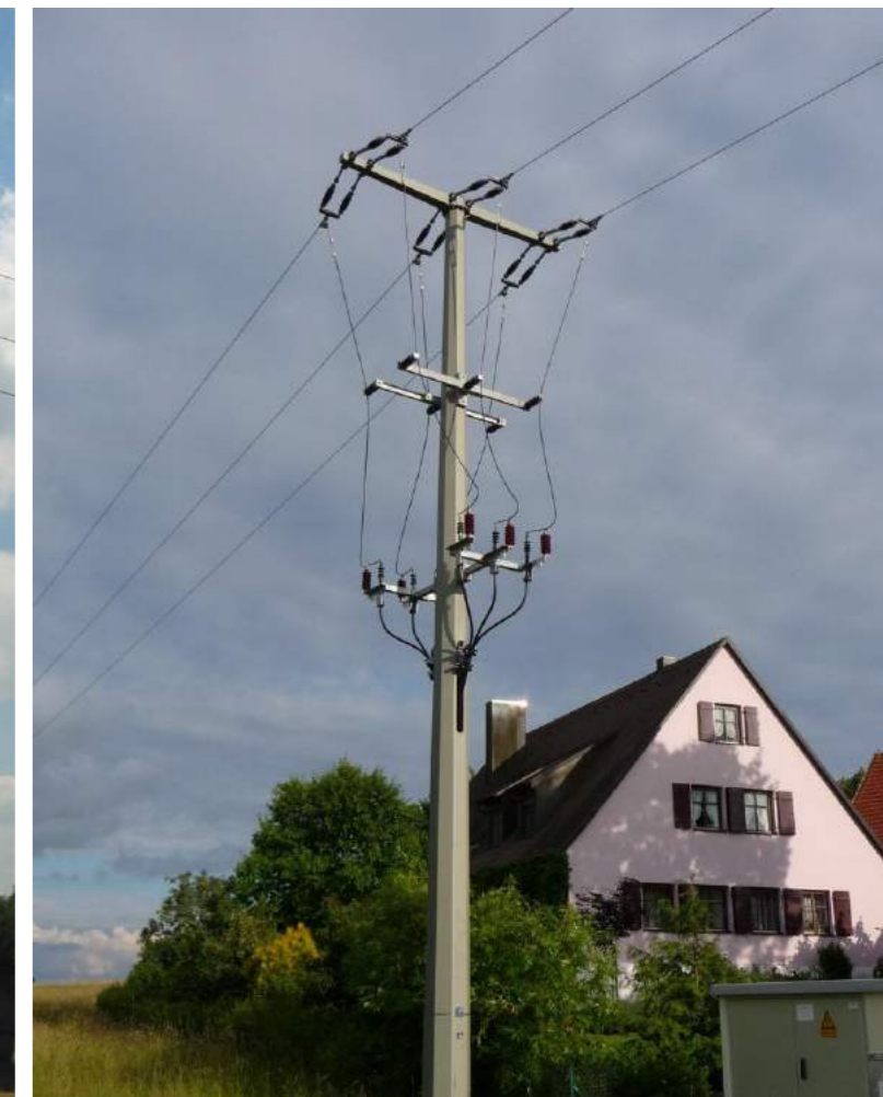
Double Cable Termination Pole
