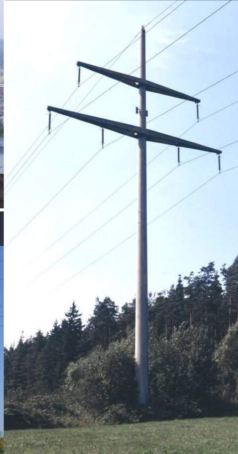
110kV Concrete Pole
