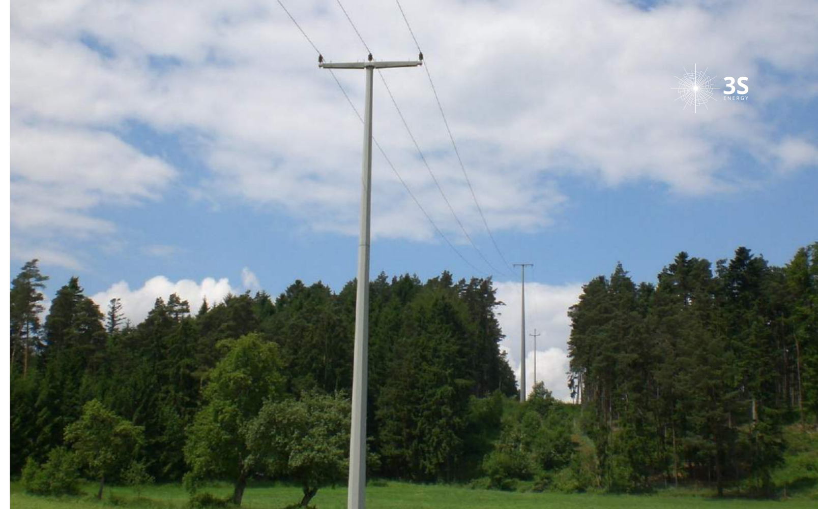
Forrest Crossing – different isolator arrangements
