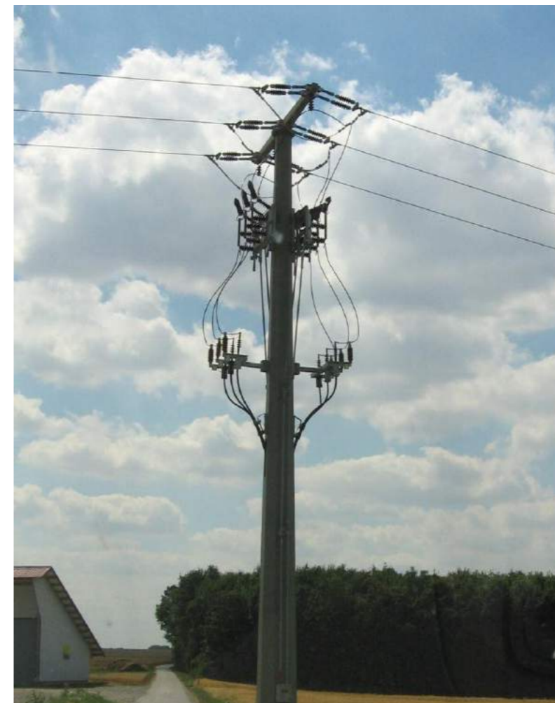
Cable termination & circuit breaker pole
